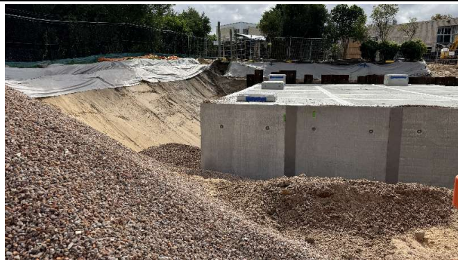
Photo 8 & 9: Northern boundary - Erosion and sediment controls (ESC) were installed along the northern boundary. At the time of inspection, the construction site surface levels were lower than the adjoining boundary, reducing the risk of off-site discharge of sediment-laden water.
