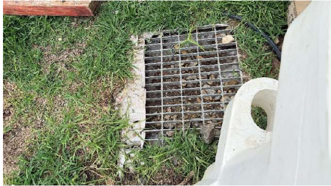
Photo 10: Northern boundary – Stormwater grates within the construction zone were protected with geofabric to minimise the ingress of sediment and rubbish into the stormwater system.
