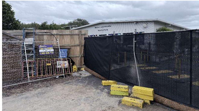
Photo 3: Northeastern corner – Early Learning Centre (ELC) located adjacent to the construction site, separated by physical hoarding and shade cloth screening.
