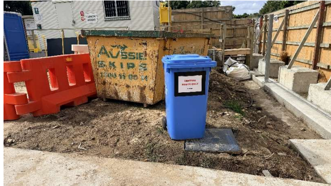
Photo 6: Western boundary - Waste skip provided for packaged wastes, with designated bins for general waste segregation.
