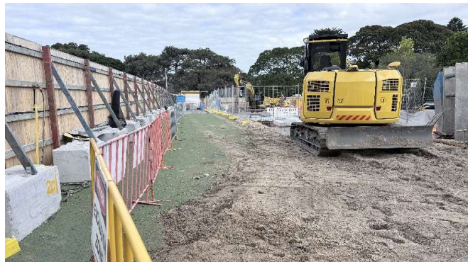
Photo 4: Southern boundary – Hoarding delineating the construction site. Astro turf was installed along the designated worker pedestrian pathway to minimise tracking and spread of sediment outside the construction zone.
