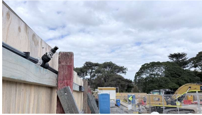
Photo 5: Southern boundary – Fixed sprinkler systems installed for dust suppression.
